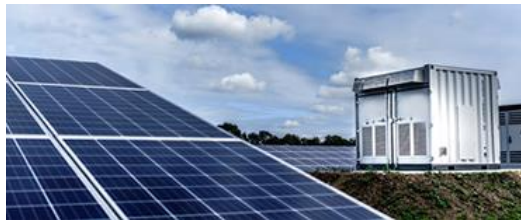
储能电池/Energy storage battery
